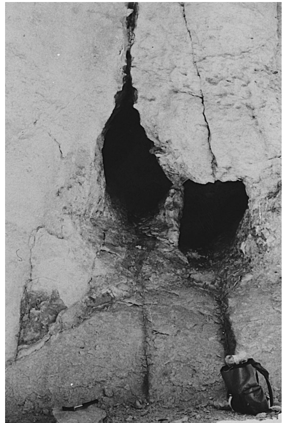
Fig. 3. Subhorizontal double shaft, developed along vertical joints and showing vertical blackish trails at the outlet, suggesting water outflow. Flaking spheroidal mantle visible below the orifices.
